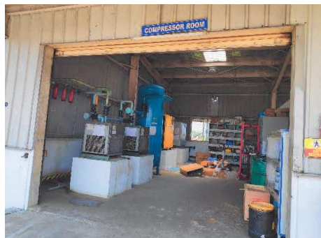
View of the compressor room
