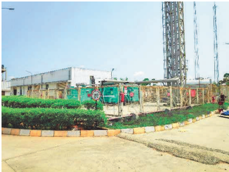
View of the DG set
