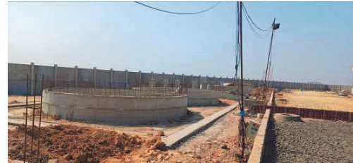
View of Modular Tank Pump Room
