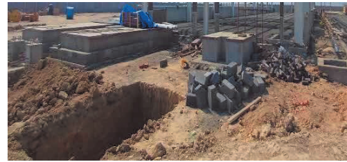
View of DG Platform & Transformer Yard
